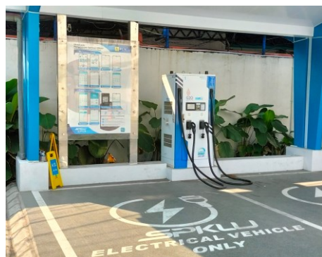
Fig. 4. One of public charging facility for 4W-EV in Bandung.
